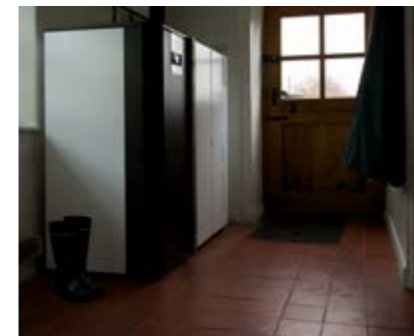
44 UTILITY WOOD PELLET BOILERS
